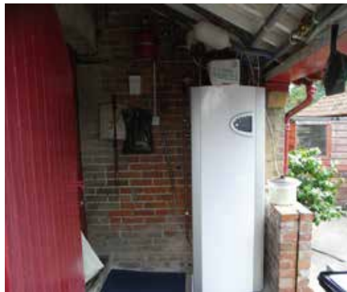
Residential ground source heat pump
